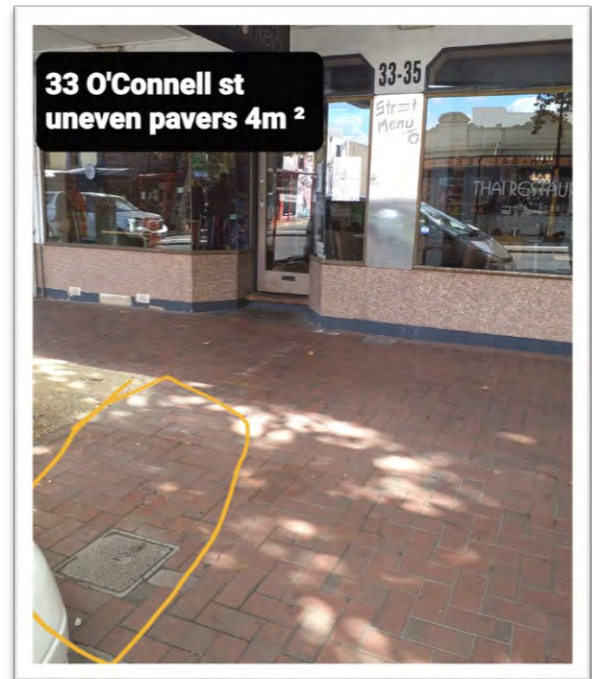
Image 36 - Area of paving requiring maintenance
