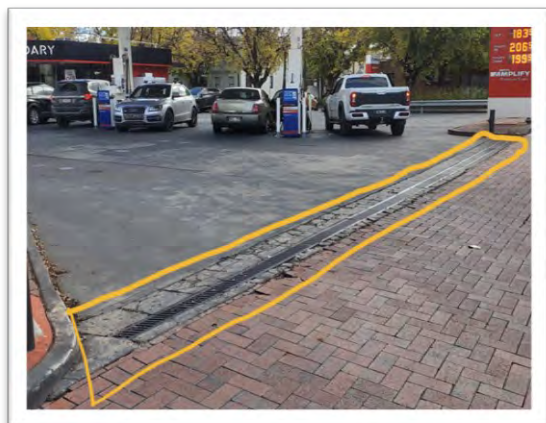
Image 53 - Damaged infrastructure 131 O'Connell Street
