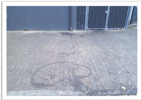
Image 31 - Oil-stained footpath requiring a deep clean - 22 O'Connell Street - side street
