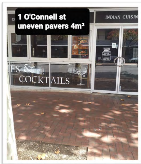
Image 35 - Area of paving requiring maintenance
