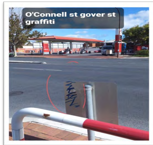
Image 27 - Graffiti identified during Condition Audit
