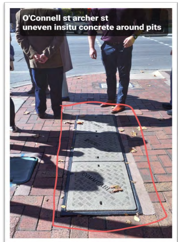
Image 37 - Area of paving requiring maintenance
