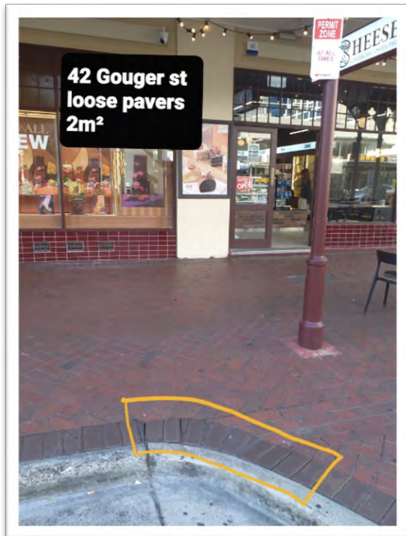
Image 3 - Loose pavers noted along back of kerb at 42 Gouger Street
