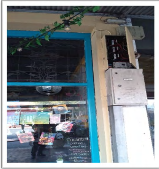
Image 15 - Missing fuse box cover
