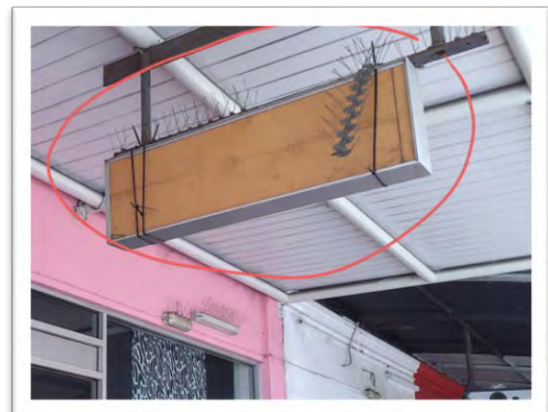
Image 55 - Anti-bird device not installed correctly.
